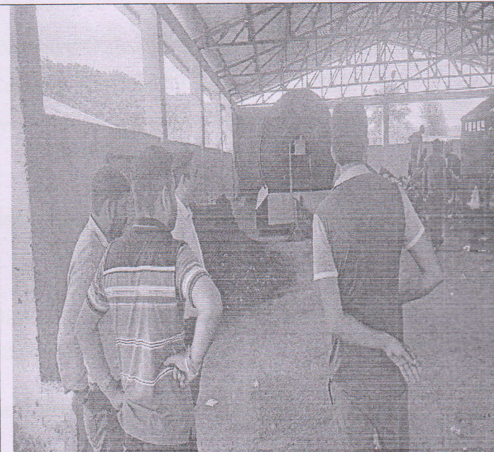
Photograph No.4 —Shows Status of Two nos. of Organic Waste Composting Machines Installed at the Site.
